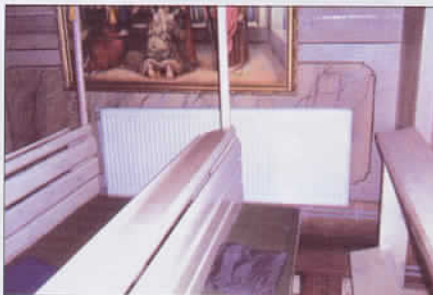
New heating system installed
